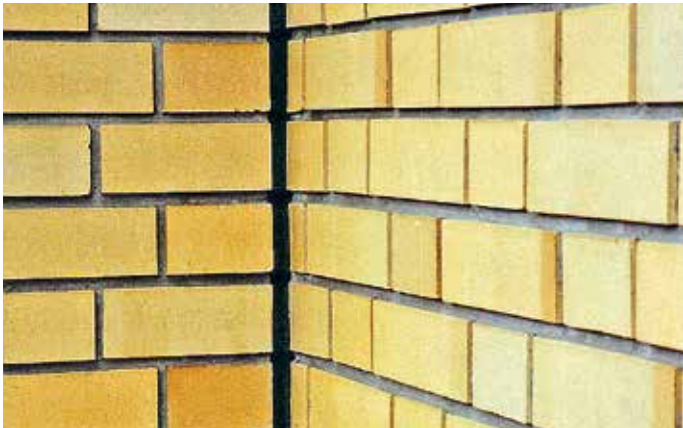
Building construction joints in accordance with DIN 18540, sealed with EGO SMP 818 in masonry construction
